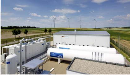
Hydrogen Storage System
