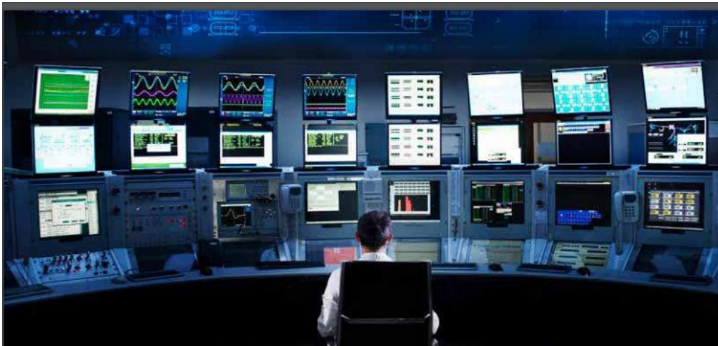
Figure 3 - Picture of control room for the power sector [5]
